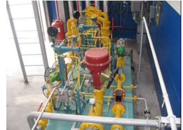
Gas fuel preparation unit
