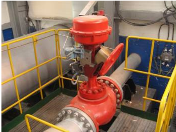
Anti-surge valve Dresser Masoneilan DN350
