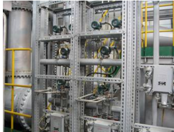
Pressure transmitters Yokogawa EJX
