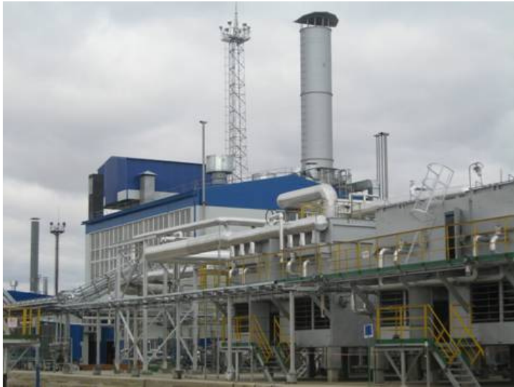
Compressor Station overview
