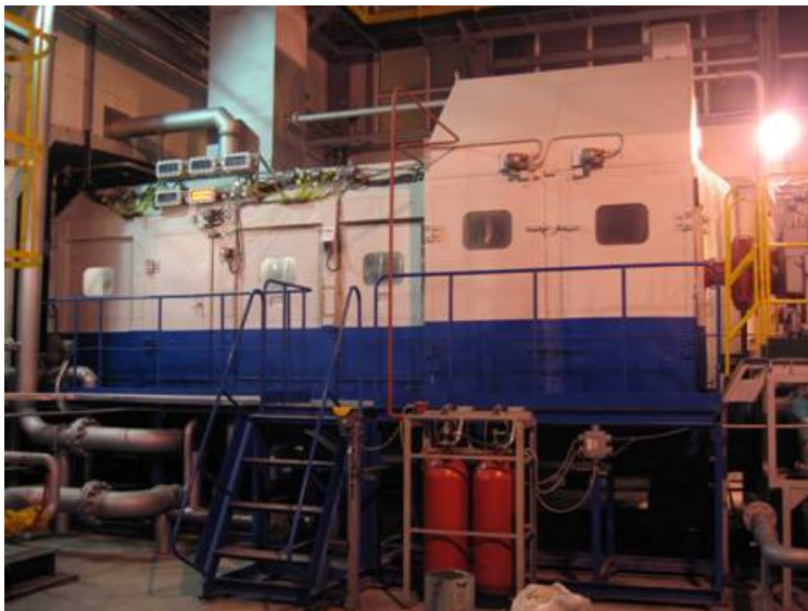
Turbine Powerplant NK-16STD (16 MWt) in protective housing
