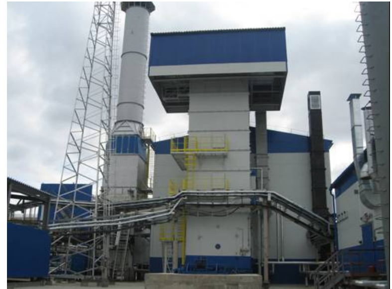
Air intake and filtering unit
