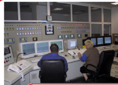
Operator Main Control Room
